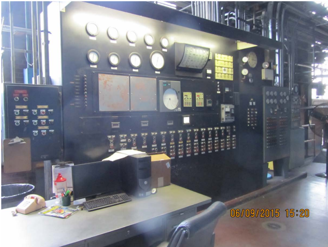
Obsolete control panel from 1947 at NIOSH campus in Pittsburgh, Pennsylvania
