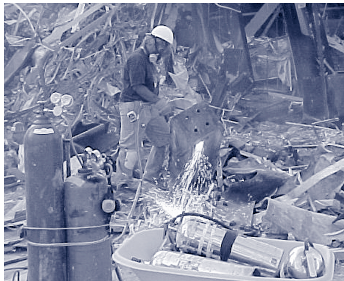
FIGURE 1. A worker clears rubble at the World Trade Center disaster site using an oxyacetylene torch
