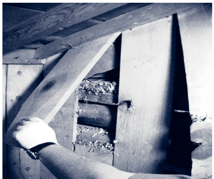
FIGURE 1. Rodent nesting material found inside the interior walls of a cabin — New Mexico, 2002
