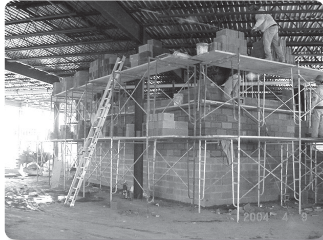
Problem: Conventional unguarded frame scaffolding
