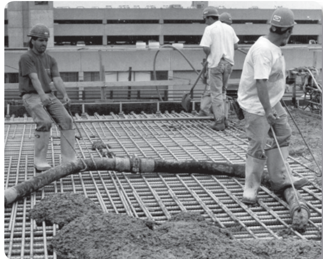
Problem: Pulling concrete hose without skid plate
