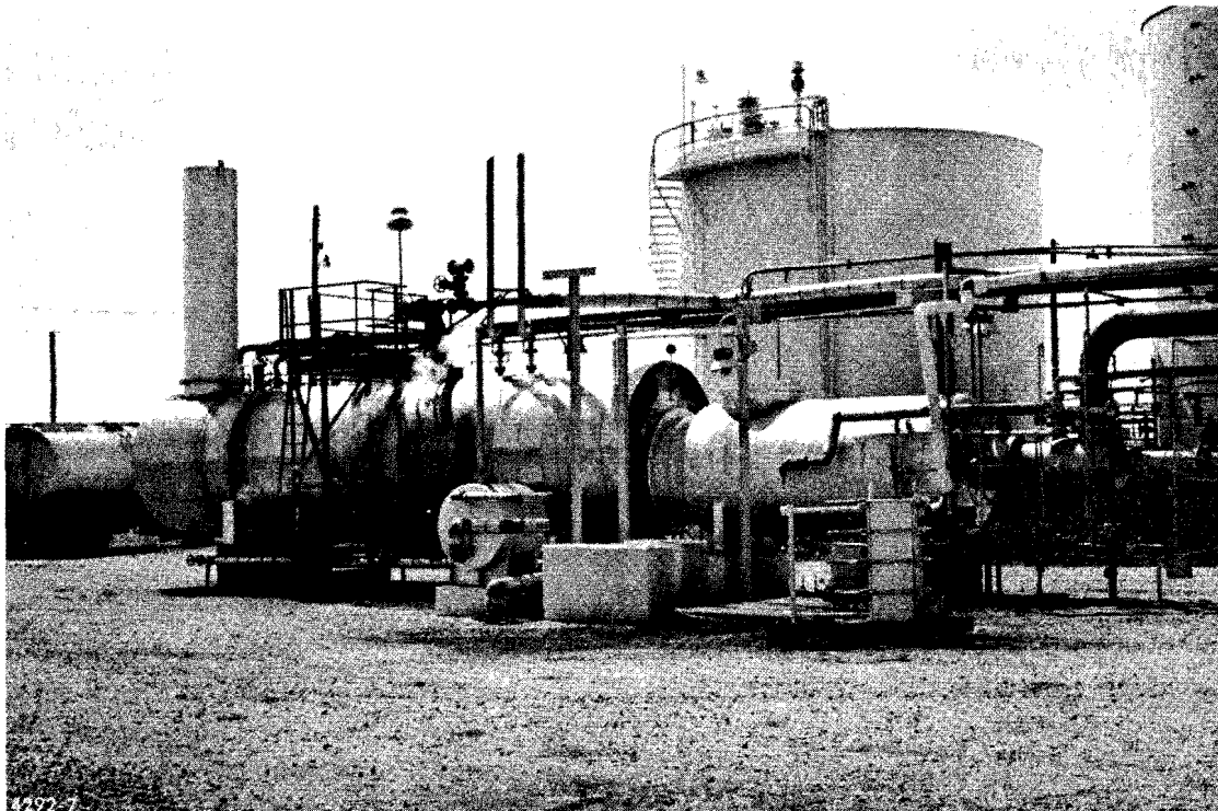
Figure 6. Incinerator for waste gas.
