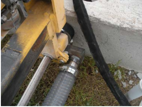
Figure 9 – Another view of the hood
