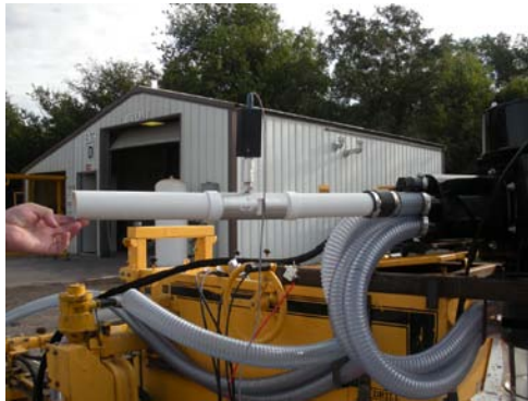
Figure 6 - Exhaust ventilation measured at collector with hose disconnected
