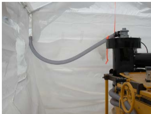
Figure 3 - The exhaust from the pneumatic fan motor was routed outside the tent
